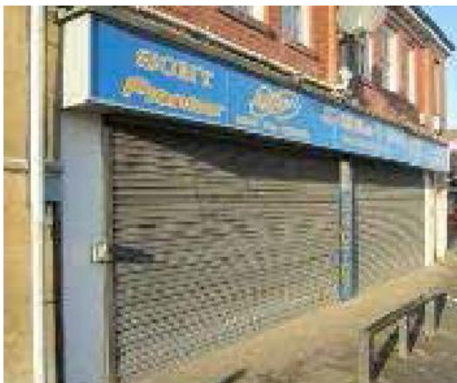
Visually harsh and unsympathetic external roller security shutters with bulky grille boxes
